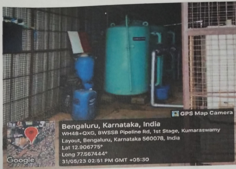
SEWAGE WATER TREATMENT PLANT
