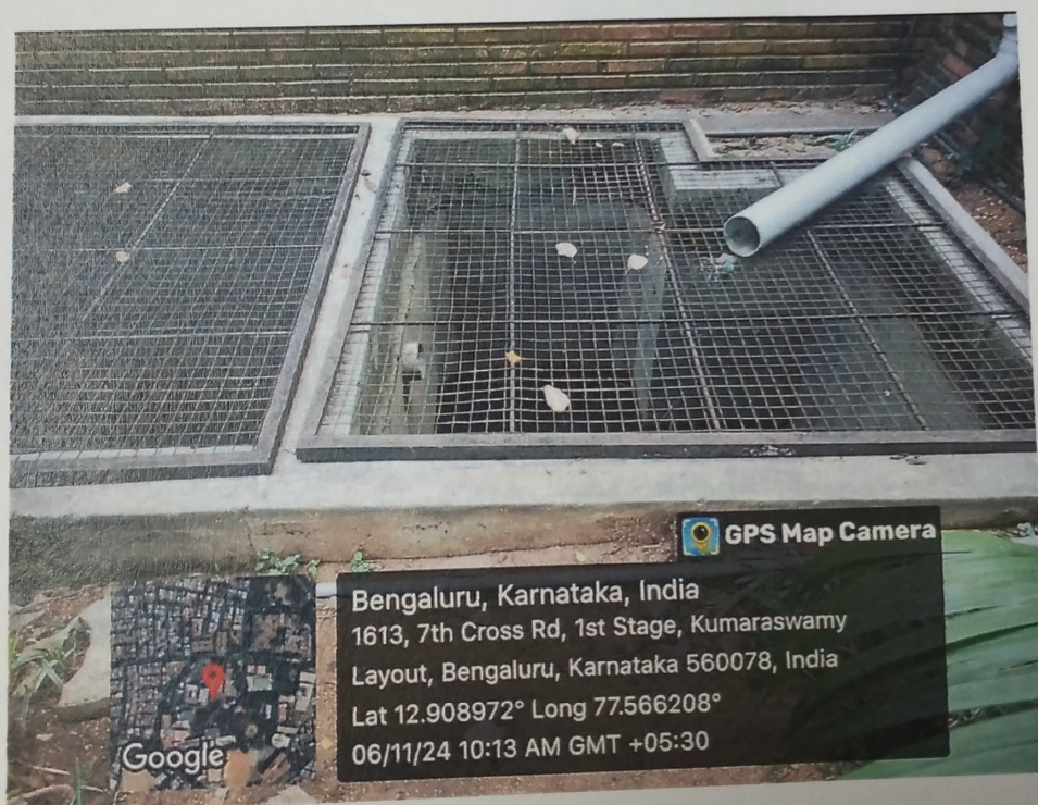
RAINWATER HARVESTING FACILITIES IN THE CAMPUS
